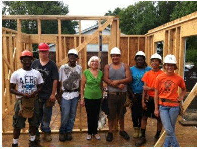
Some of our 2013 construction students at the build site with State Representative Naomi Jakobsson
